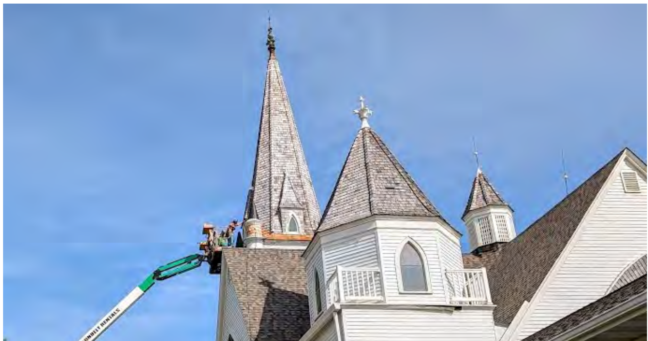
Vang Lutheran Church, Dennison, Minn., is restoring its iconic steeple as part of a larger renovation project to preserve the church's historic building. The church received a $100,000 matching grant for its preservation project. Photo: Church Property Resource Hub.
