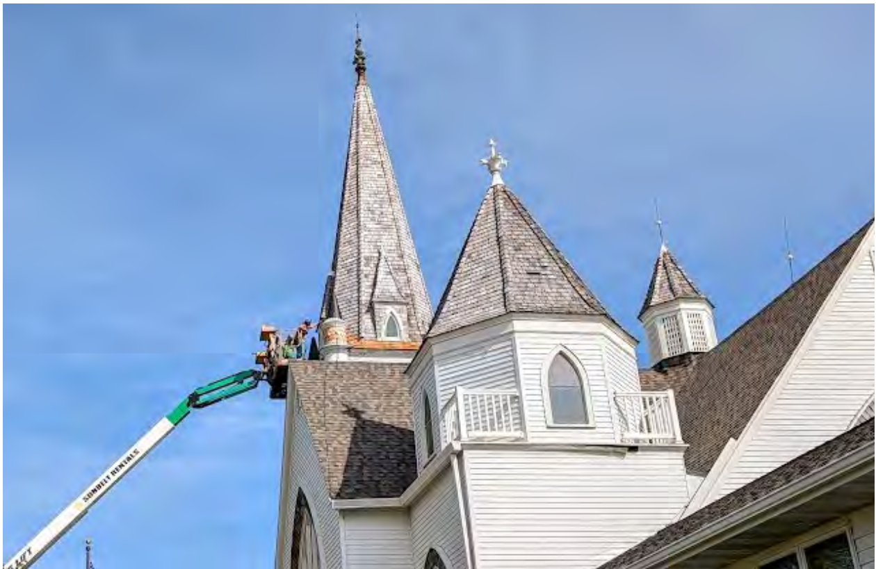
Vang Lutheran Church, Dennison, Minn., is restoring its iconic steeple as part of a larger renovation project to preserve the church's historic building. The church received a $100,000 matching grant for its preservation project. Photo: Church Property Resource Hub.
